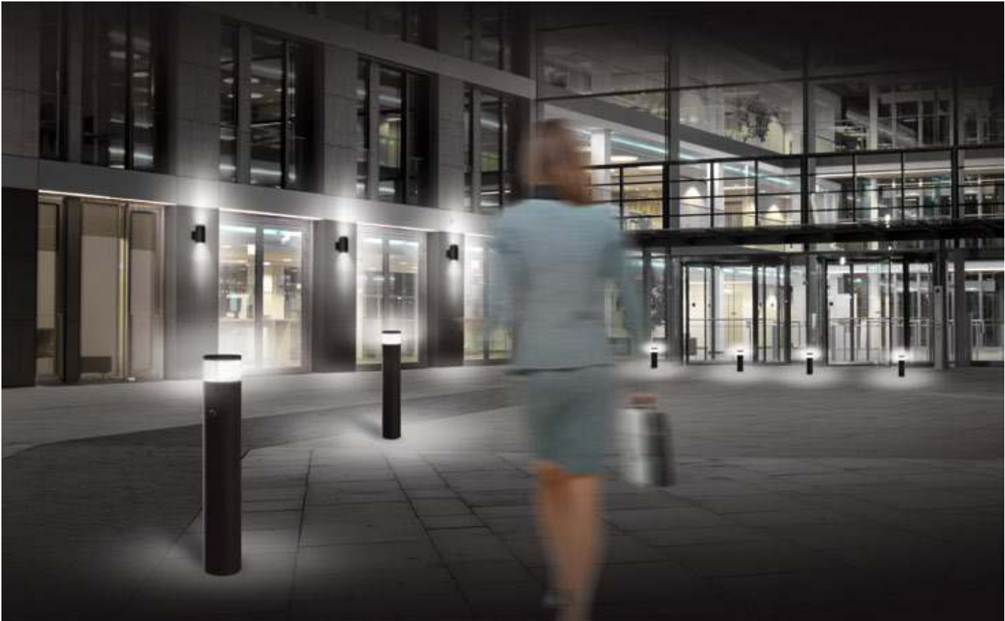
Individual control of various end devices using an intelligent DALI network.
