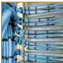
Data Cabinet Installations
